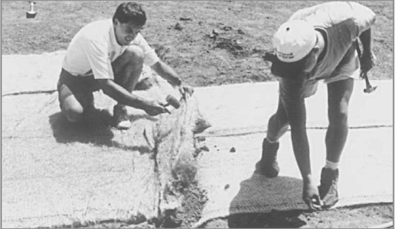
Figure 6.30 Follow manufacturer's recommendations to successfully install erosion control blankets or matting. The manufacturer of this high velocity blanket called for stapling every two feet and a check slot wherever two sections were joined. This blanket was used to protect soil and establish grass in a waterway on the August Busch Memorial Conservation Area
