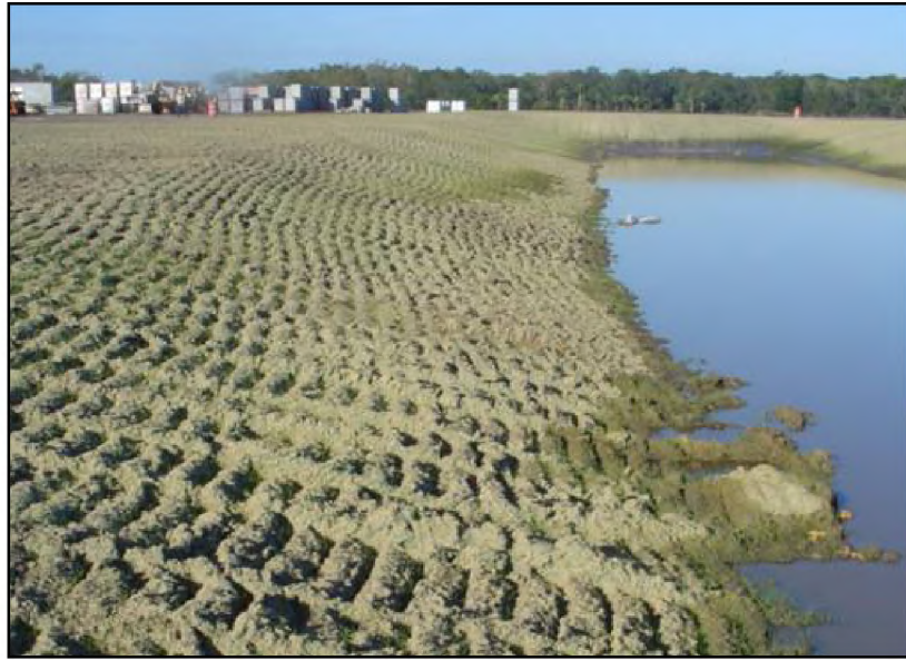
Figure 6.15 Track walking with a dozer up and down the slope provides horizontal grooves to reduce stormwater flow volumes and velocity therefore reduces potential for erosion of the slope. Source: ABC's of BMP's, LLC
