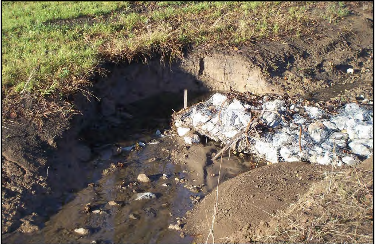
Figure 2.3 The improperly installed check dam created significant bank erosion. Source: ABC's of BMP's LLC
