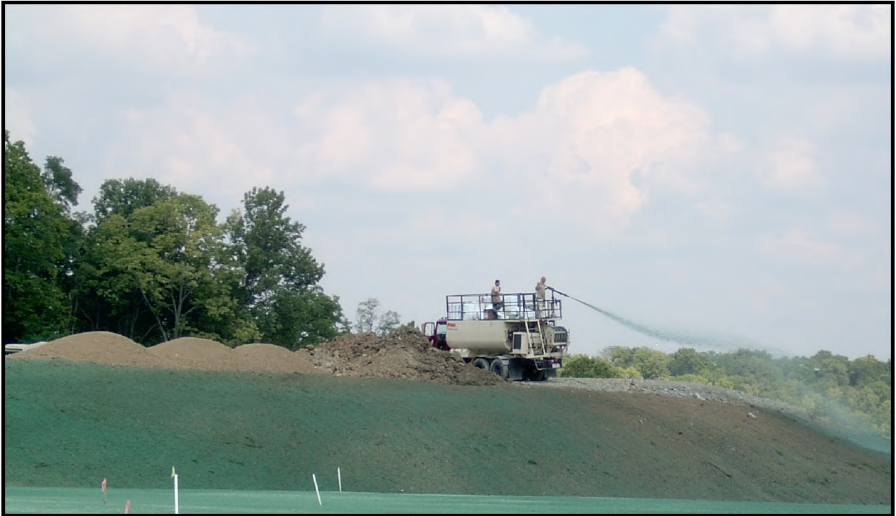
Figure 6.26: Hydroseeding over mat armoring on a steep slope to promote vegetation growth and prevent erosion. Source: Florida Erosion and Sediment Control Designer and Reviewer Manual , June 2007
