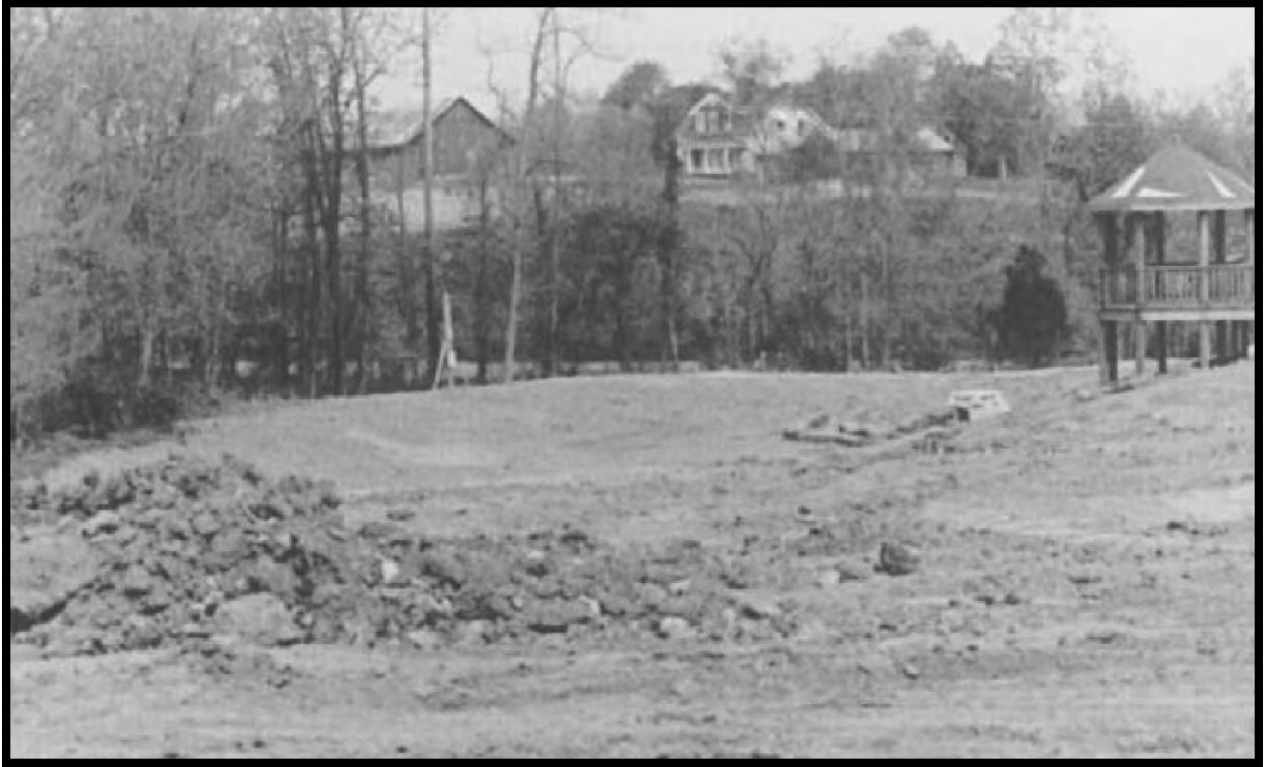
Figure 6.55 An unfinished temporary diversion routes sediment-laden storm water to a sediment basin. Temporary diversions should be shaped and protected with a turf reinforcement mat or rock. Establish permanent vegetation if the diversion will be used for one year or more. Source: K. Grimes, Soil and Water Conservation District, St. Charles Co.
